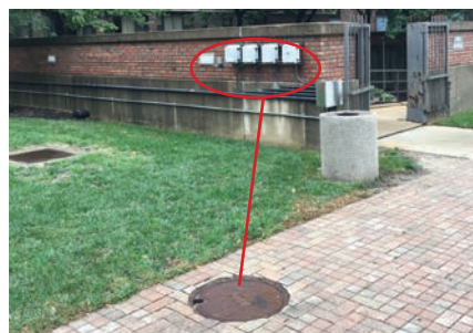
Unit can be mounted externally (remote monitoring)
