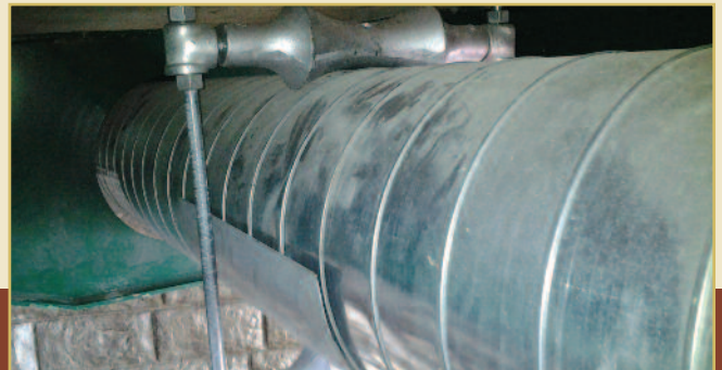
The Rovanco product does not require any special guides or saddles. This picture shows the piping installed under a bridge.
